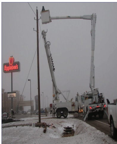
Crews work to restore power in Altus, Oklahoma as a result of a winter storm.
